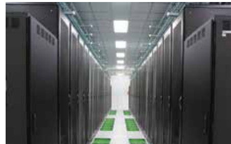
IT infrastructure (High-density Racks)
