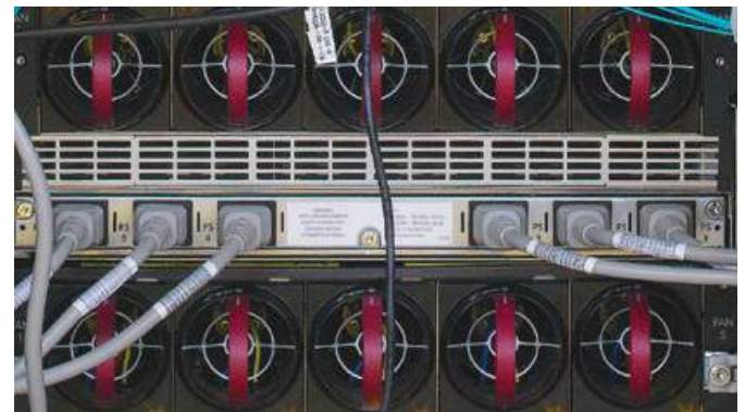
Typical server with multiple power inputs powered by two ePDUs
