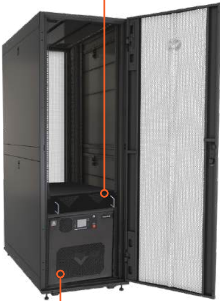
Battery Module (3U)
